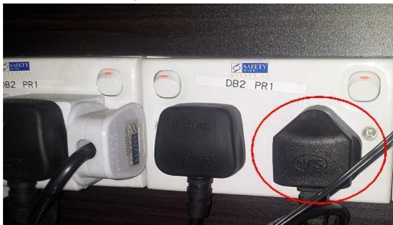
Check power cable and sockets
