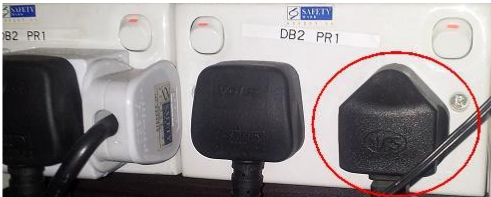
Check power cable or sockets
